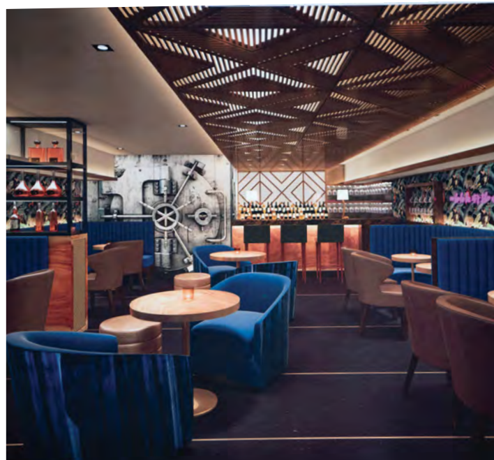
The company owned by Joseph Colaluca '09, '15G is renovating 383 Admiral Street, the former home of Club Eagles and Clubbies, into a restaurant. The building will have three floors of dining, including a basement speakeasy.
