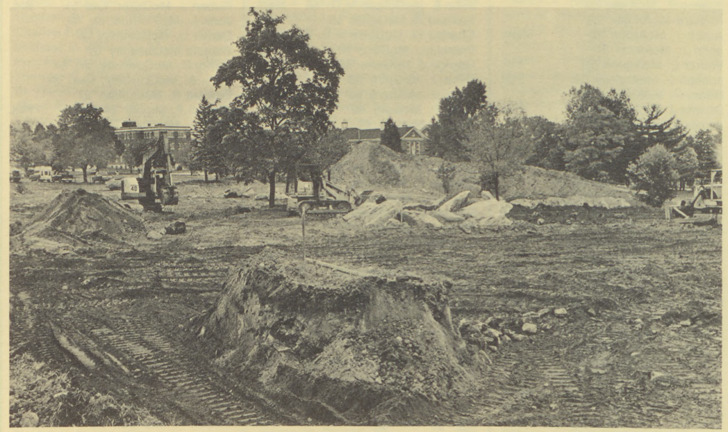
By October, 1975, work was well underway on the multi-purpose field for soccer, football and field hockey. In addition two intramural softball fields were constructed.
