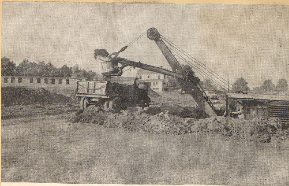
"FILL 'ER UP" says the truck driver as excavating for the proposed new gymnasium continues. The site is the rear of Donnelly Hall where initial preparations for the new athletic plant are being made. The first phase of operations will consist of excavating for the foundation before the frost sets in. Actual construction is not expected to begin before spring.
